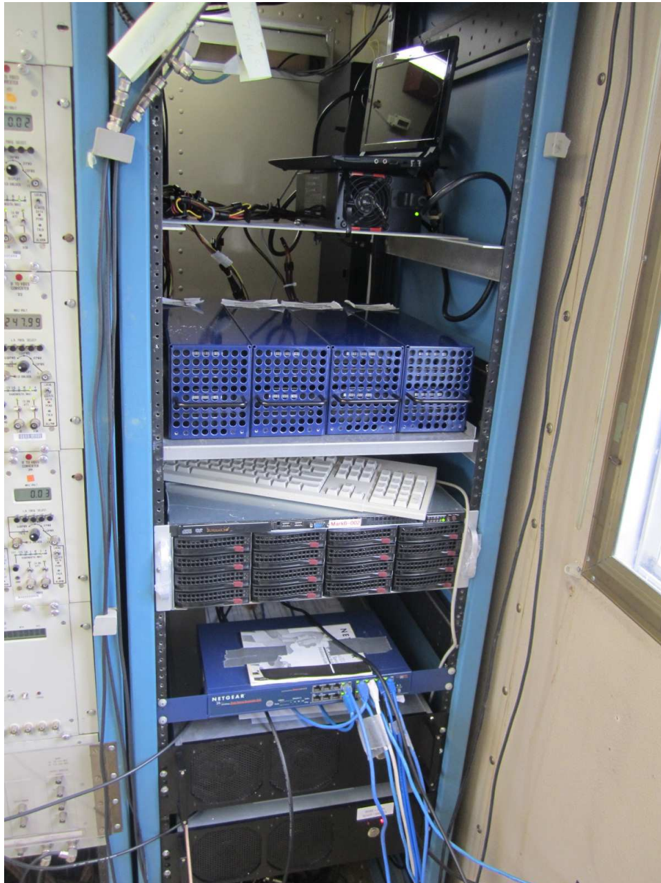
Figure 21: The two RDBE-S units were installed at the bottom of the available rack at GGAO. The Mark6 recorder is above the network switch (the disk bays are empty). Above the Mark6 are 4 prototype disk packs containing 32 disks.
